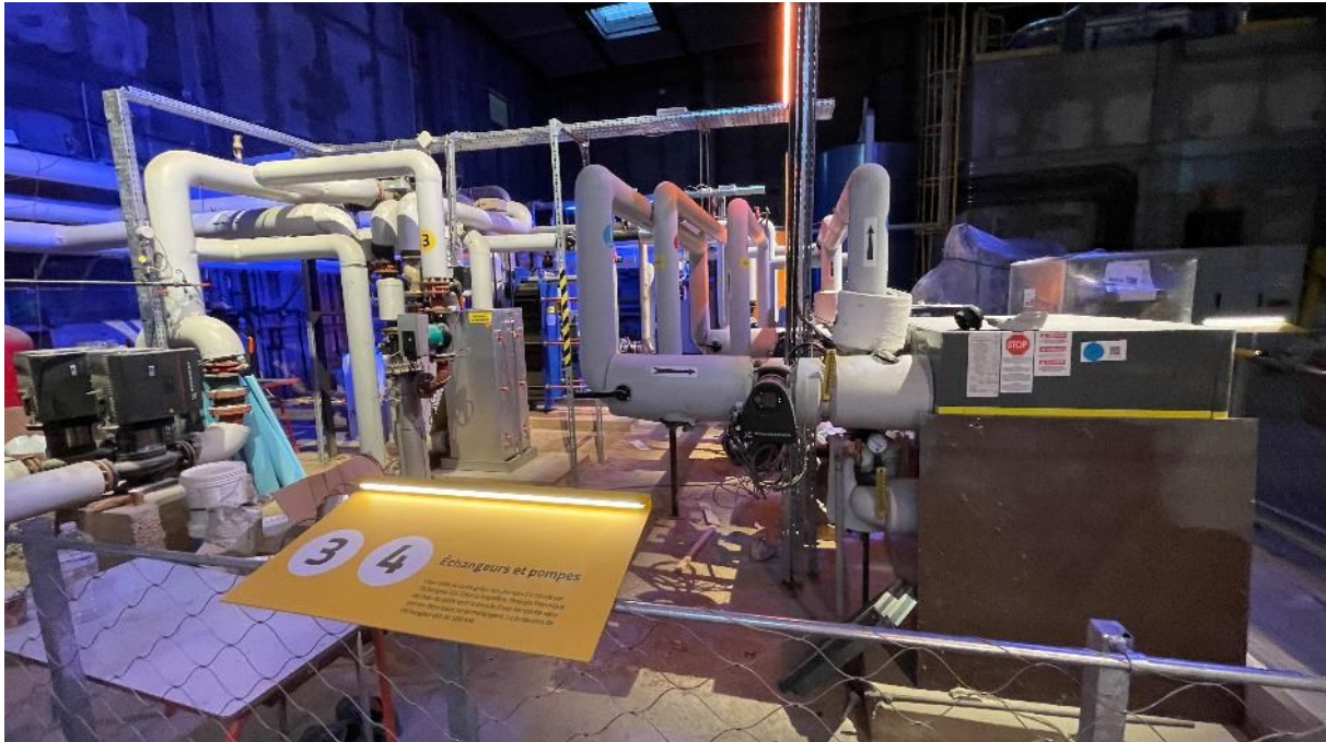
Figure 16: view of the substation with the integrated dynamic lighting and explanatory booth detail. Source: ENSOL.
